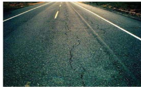
Low fatigue cracking
