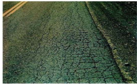
High Fatigue Cracking
